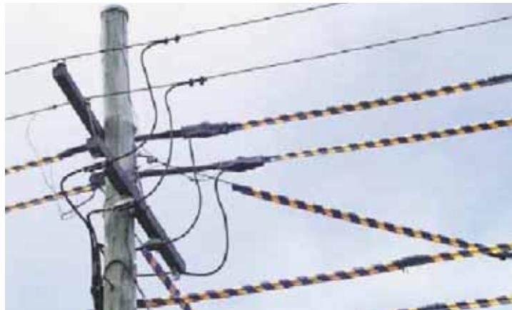
Figure 16 – Tiger tails fitted to overhead power lines
