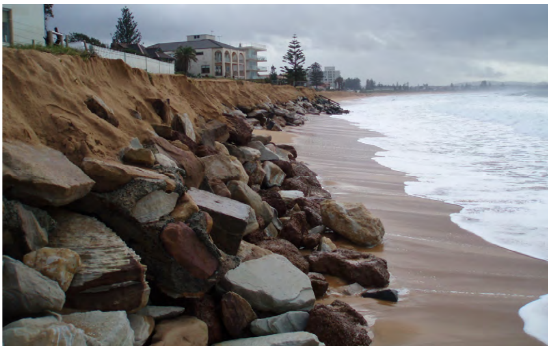
Figure 5: Exposed rock protection between Stuart Street and Wetherill Street, 17 June 2007
