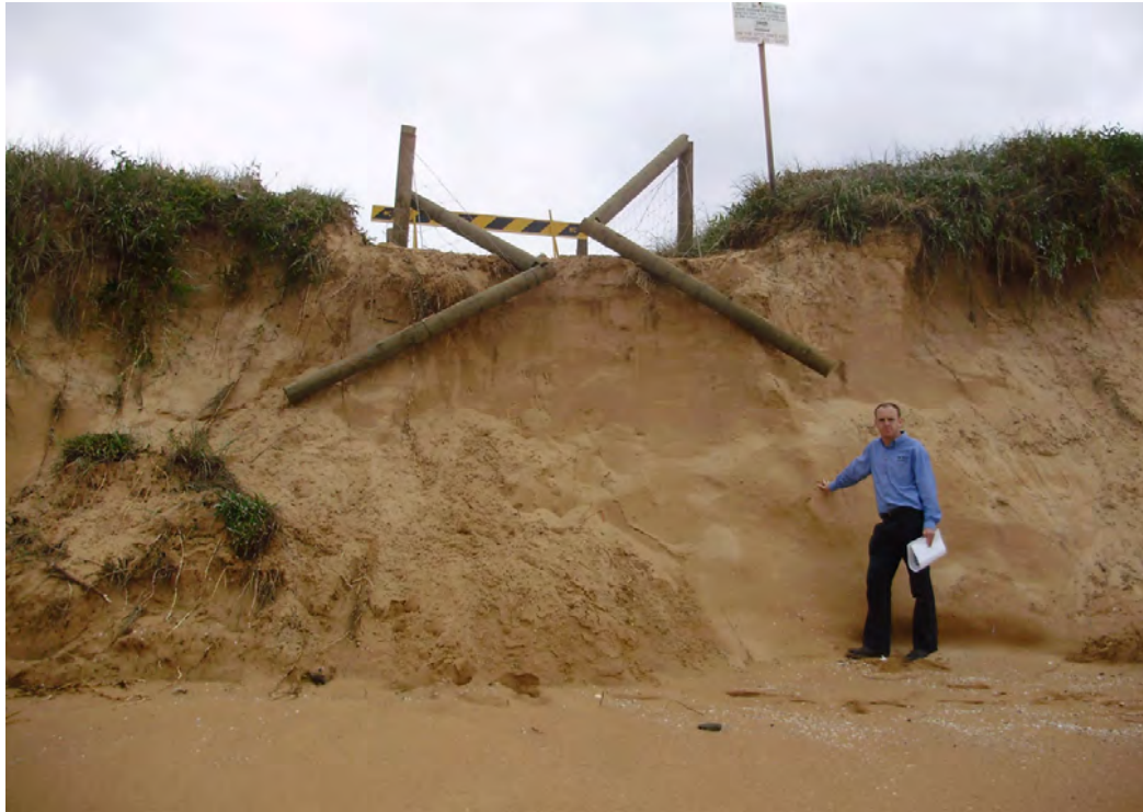
Figure 19: Damaged beach accessway at North Narrabeen Beach in May 2009
