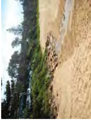
3. Scour at stormwater drain and weed growth over embankment, Marine Parade MacMasters Beach, 3 April 2014
