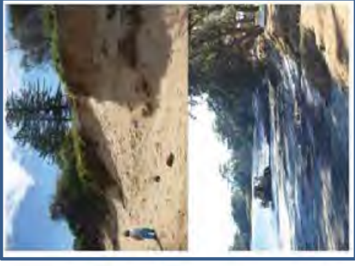
Beach scraping to repair eroded beach escarpment and repair of beach accessways
