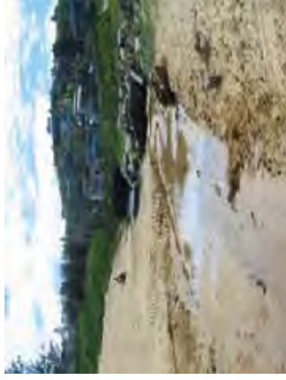
7. Scour at stormwater drain and creek entrance, near Copacabana surf club, 5 October 2010
