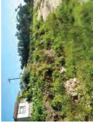
2. Ad-hoc erosion protection and embankment erosion along Berrima Crescent properties, south end of beach, 3 April 2014
