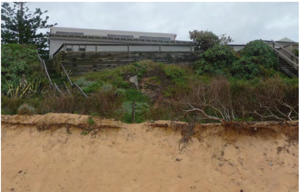
Figure 20: Timber retaining wall and rubble at 3 Calais Road, 24 November 2011
