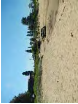
6. Scour at stormwater outlet, Umina SLSC 3 April 2014
