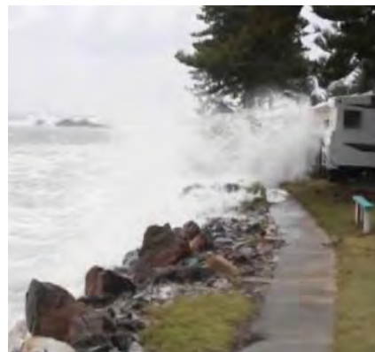
Plate 2 Wave overtopping at southern end of caravan park 25/12/2011 (Mr Mark Cameron)
