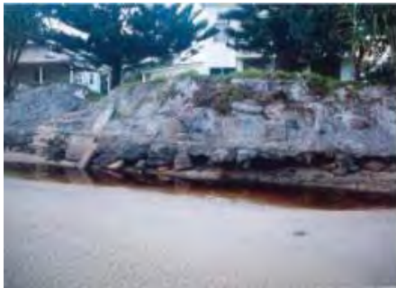
Plate 9 scour at the revetment toe 13 th February, 2002 (source: CVC)
