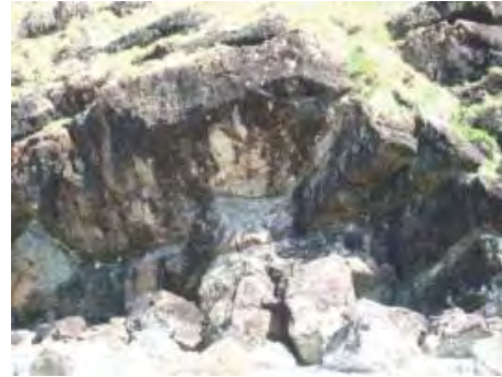
Plate 8 Crest Fretting & Block Toppling Point
