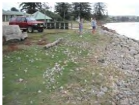
Plate 4 Rock & debris near boatramp from revetment overtopping 6/6/2012 (CVC)
