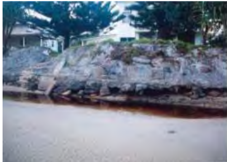
Plate 3 scour at the revetment toe (13/2/2002 source: CVC )
