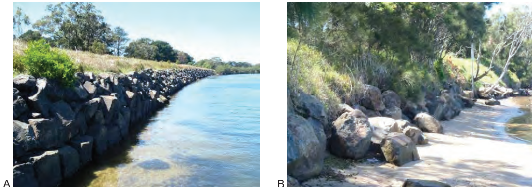
Figure 31: Riverside Drive erosion controls
