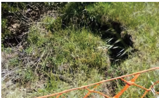
Site 9 - Riverside Drive stormwater scour
