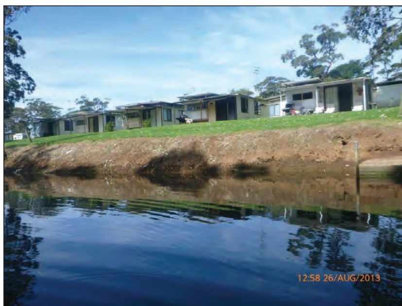
Figure 11(c): Areas of exposed bank in Blue Angle Creek
