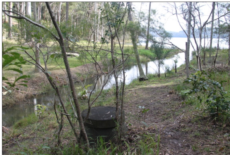
Low-lying manhole located next to creek entering Smiths Lake
