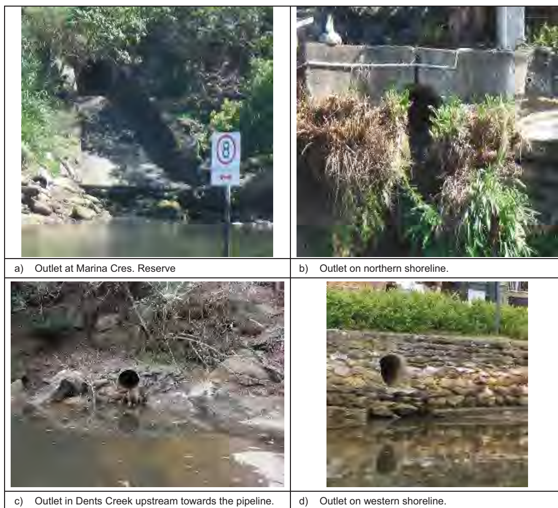
Figure 6-5: Council Stormwater Outlets
