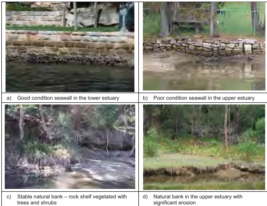
Figure ES-3: Bank condition assessment photographs
