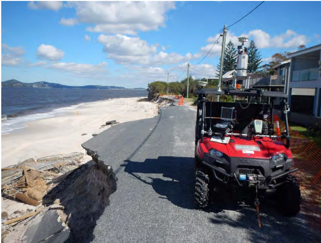
Figure A9 Road damaged by coastal erosion, Jimmy's Beach, Hawkes Nest (Photo: P Davies/OEH)
