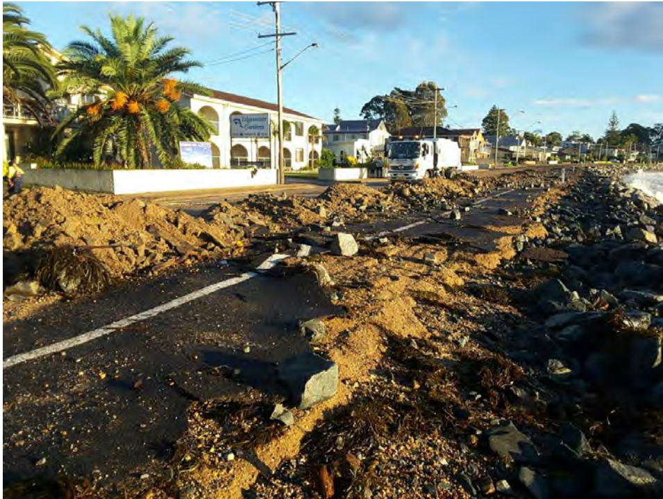
Figure B2.22 Damage to the foreshore at Casey's beach creates risks to public safety (Photo: G Armstrong/Eurobodalla Shire Council)
