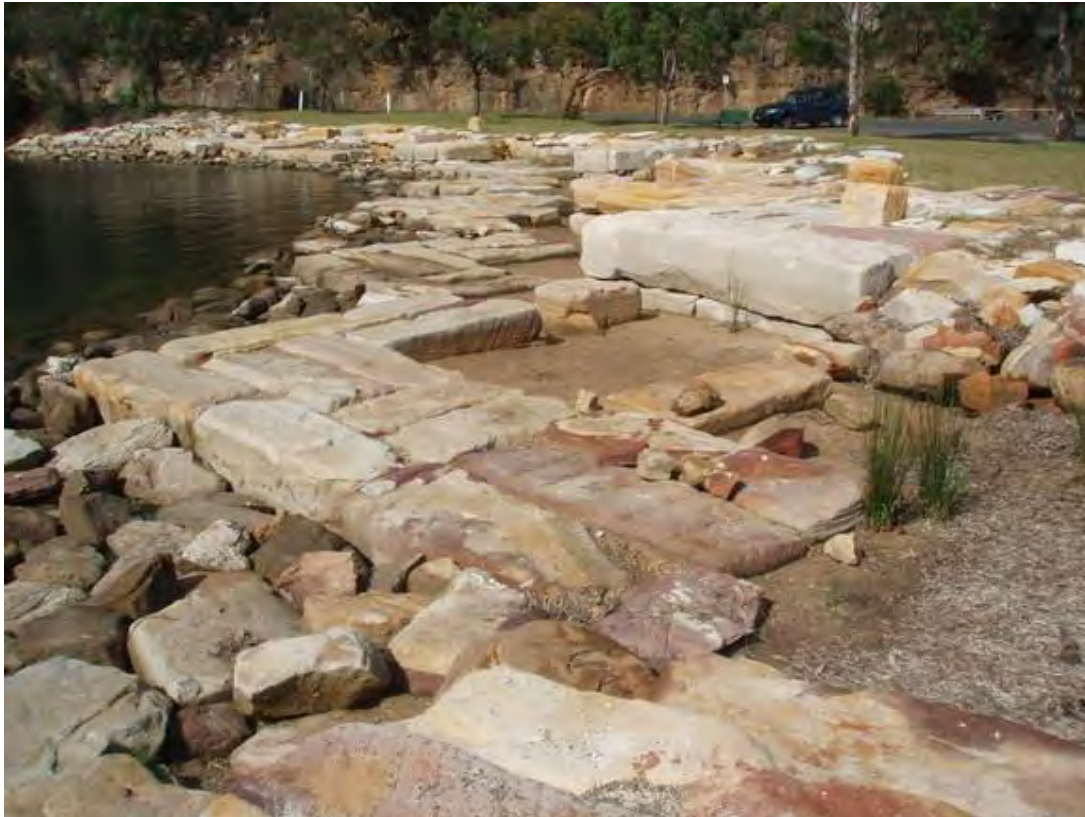
Figure B3.18 Environmentally friendly seawall made with sandstone blocks at Bobbin Head, Cowan Creek, Hawkesbury River estuary (Photo: D Wiecek/OEH)
