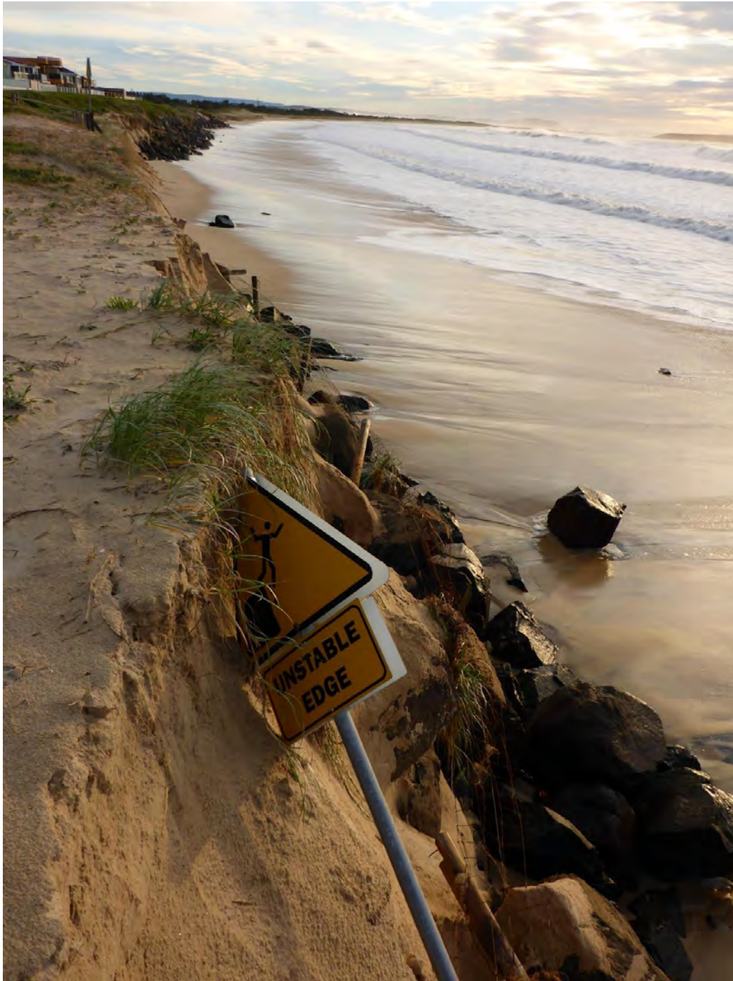
Figure B2.7 Storm damage to Warilla seawall, including loss of access control fencing and safety signage (Photo: D Wiecek/OEH)
