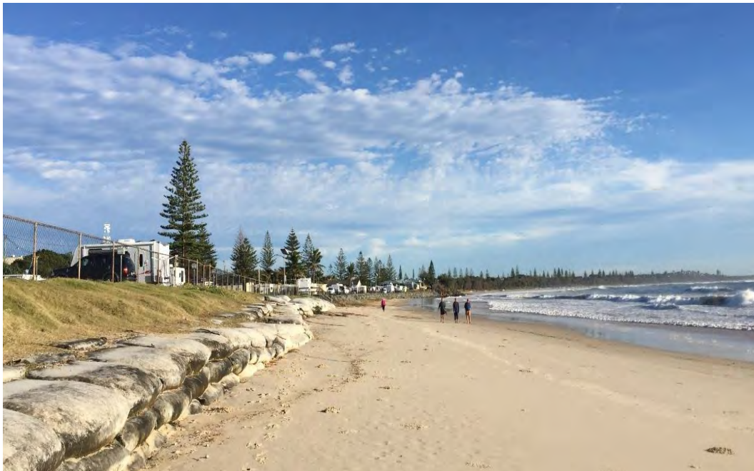
Figure B3.13 Geotextile sandbag wall, Kingscliff (Photo: M Daley/OEH)
