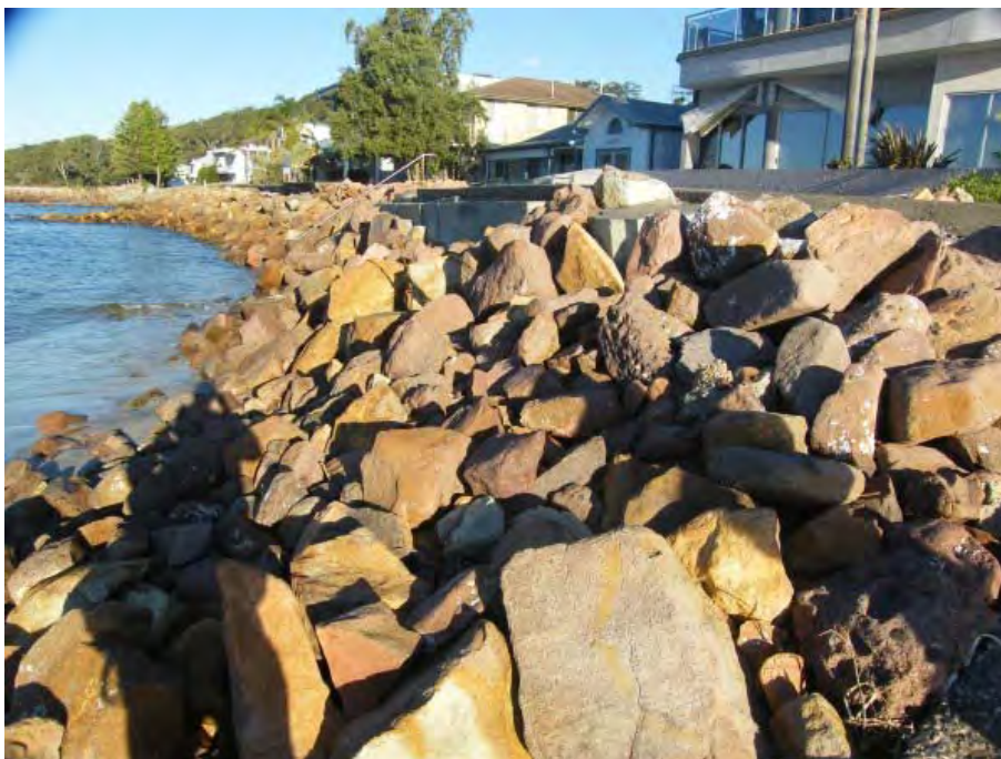
Figure 12 Western end of Precinct 5. A vertical concrete block wall has been constructed in the centre but this precinct is predominantly tipped rock. Little or no sandy beach remains, even at low tide. The public access through Precinct 5 is compromised and wave overtopping during storms is resulting in damage and inundation of property landward of the wall.
