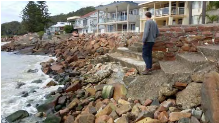
Figure 14 Eastern end of Precinct 5. Sections of the wall have undersized armour, grouted stones and various access stairs and ramps across them. Precinct 5 is the most exposed section of the foreshore and the protection provided is poor for the level of exposure. Photo Source: D Wainwright, 12 th May 2015
