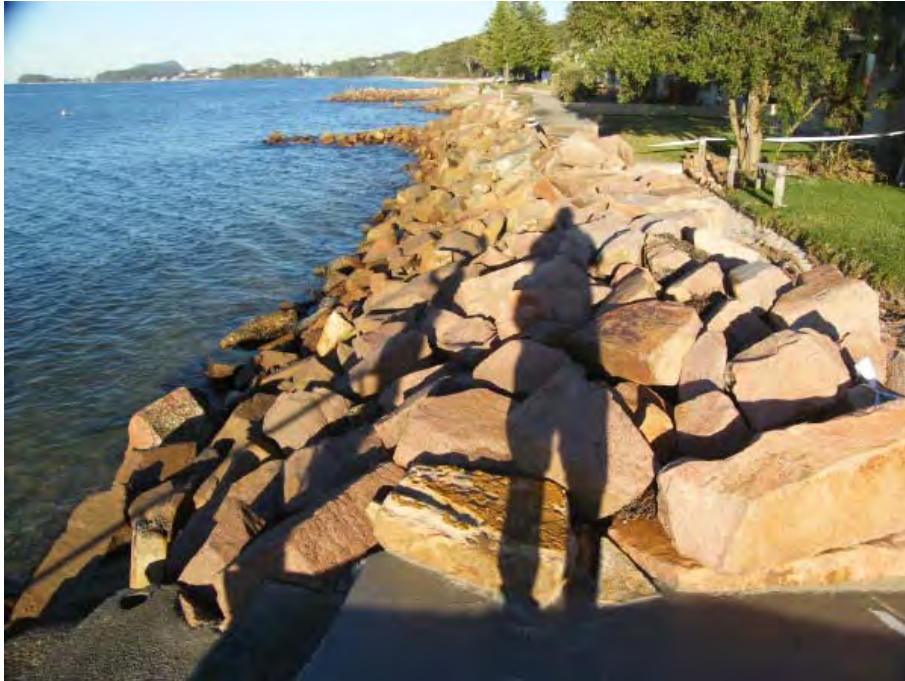
Figure 13 Much of the rock wall along Precinct 5 comprises substantial sized stone at a flatter slope. This is the most exposed section of the study area receiving ocean swells entering the Port during storms. At the time of inspection damage to the wall including loss of armour from the face and crest was observed. Scour holes under slabs and through the wall from overtopping was evident at a number of locations. The alongshore access was closed (SES tapes) along several sections. Photo Source: D Lord, 8 th May 2015
