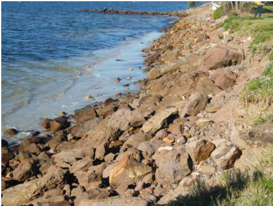
Figure 10 Precinct 4 looking east along the revetment face from the western groyne to the next groyne east. Rock armour sizes along this section are variable with significant slumping and loss of armour near the crest, exposing the erodible bank behind. The accreted sand fillet is visible in the lower left hand corner of the photo
