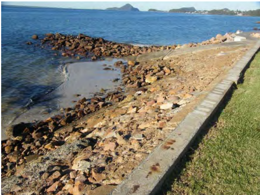
Figure 11 Eastern end of Precinct 4. A boat ramp is located west of the groyne. Rock armour has been grouted to form a smooth wall. The rock groyne has slumped and is too short and low to anchor the beach or provide significant protection. A concrete apron can be seen beyond the groyne in Precinct 5. Photo Source: D Lord, 8 th May 2015
