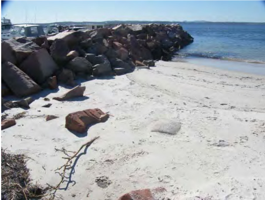
Figure 2 Western end of Precinct 1. Sand accretion against the Anchorage marina wall is burying stormwater outlets. Photo Source: D Lord, 8 th May 2015
