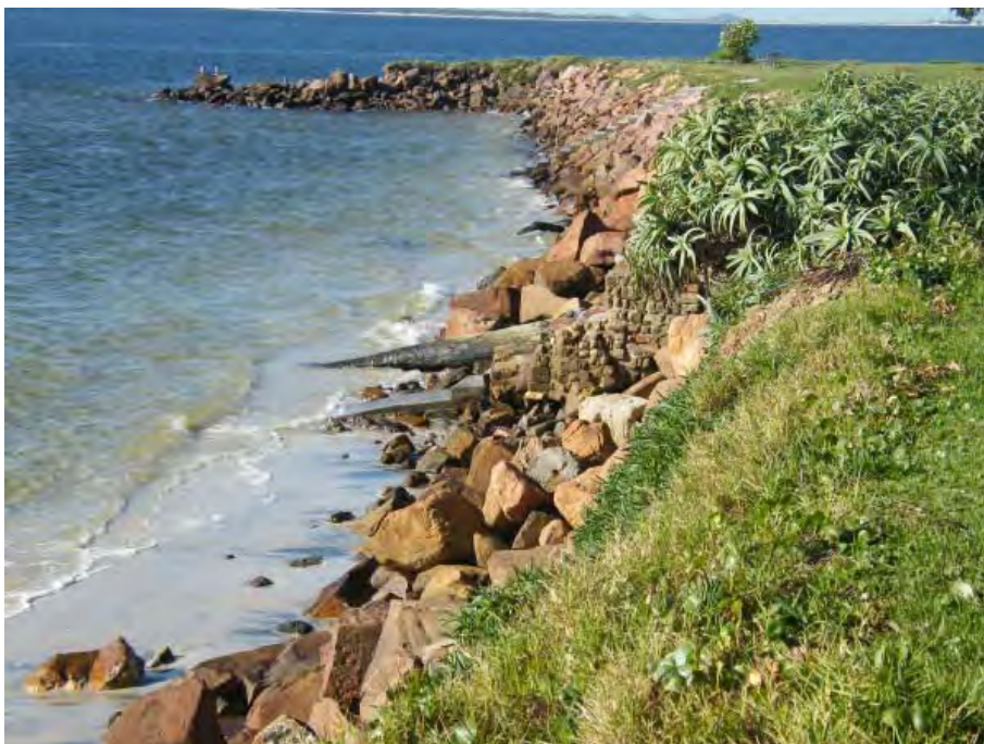
Figure 8 Precinct 3 looking east to the western groyne. Various access stairs of differing design cross the revetment. The wall is generally steep, with some slumping and loss of armour near the crest, exposing the erodible bank behind. Armour stone size is variable. The western groyne and Port Stephens entrance are at the top of the photo. Photo Source: D Lord, 8 th May 2015
