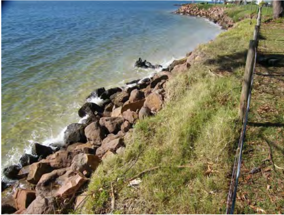
Figure 7 Precinct 3 eastern end Conroy Park. Rock protection has been placed along this section of the foreshore to the western most groyne. Photo Source: D Lord, 8 th May 2015
