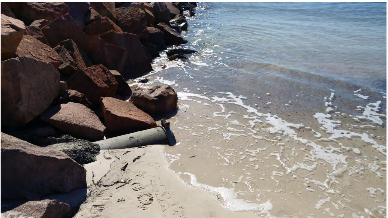
Photo 5 - Outfall 5, partially blocked with flap valve removed.
