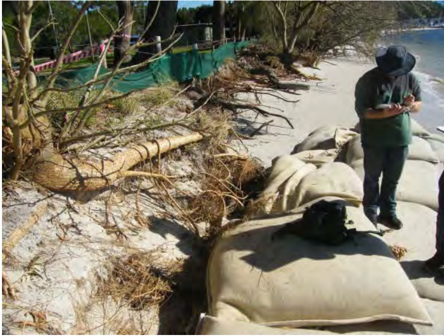
Figure 6 Precinct 2 eastern end. Geotextile containers have been employed for emergency beach protection along the eastern end of Conroy Park. Increased erosion west of the end of the protection is evident. Additional containers have been placed to extend the wall since this photo. There is little sandy beach width remaining at this location and no beach at mid to high tides. Access to the beach from the park has been affected.
