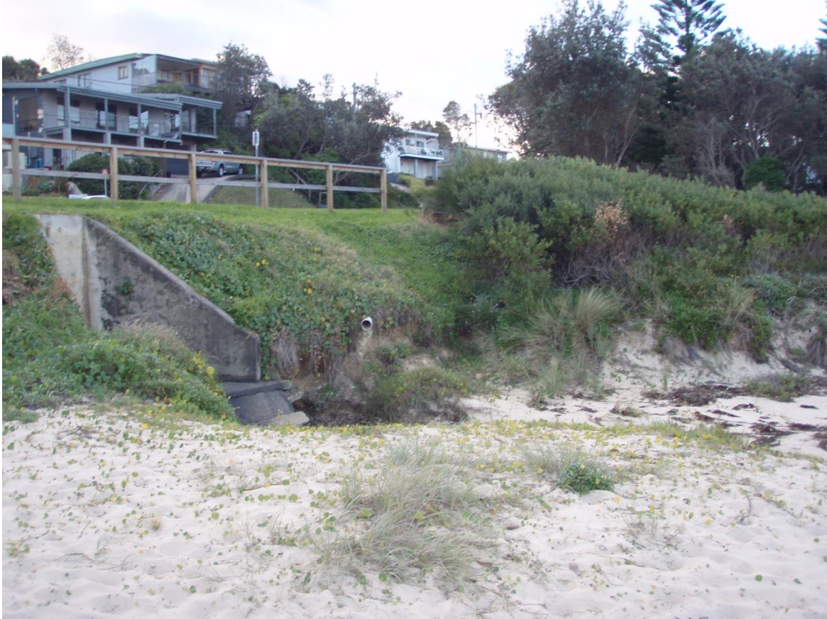
Figure 8 – Stormwater outlet at Mitchell Parade illustrating beach scour and exposure of adjacent roadway to wave inundation and erosion.
